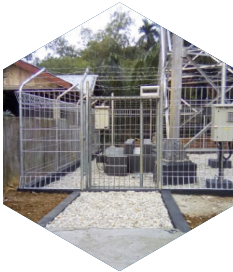
TOWER SITE & FENCING
